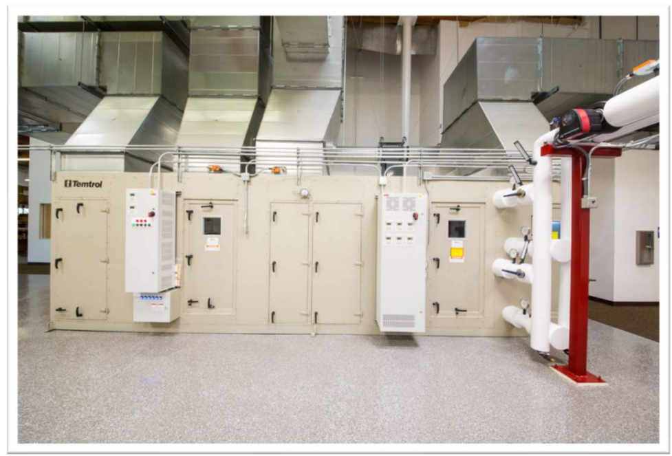
Air Handling Units
