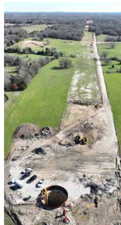
PL19TUN Open Cut ROW Restoration From Cedar Creek Tunnel to Stream A
